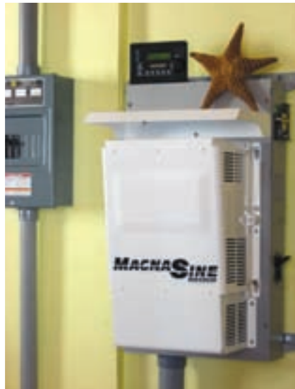
As the PV array expanded, so did the Barkers' power center. Although some of their primary loads are DC, three inverters (left and below) also convert the PV array's output for standard AC appliances.
